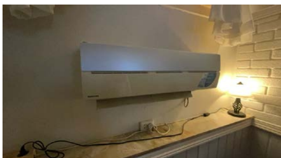
Varmepumpe, innvendig aggregat.
