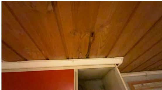
Fuktmerker i himling.
